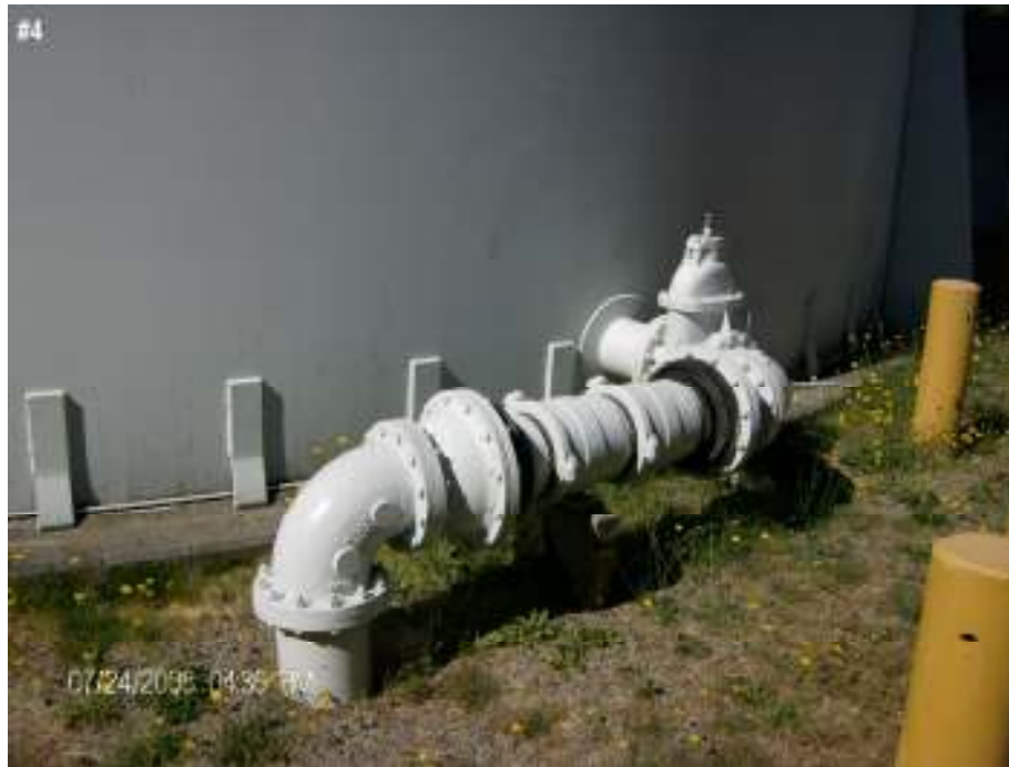
Photograph 4: View of above-ground flexible fitting retrofit
