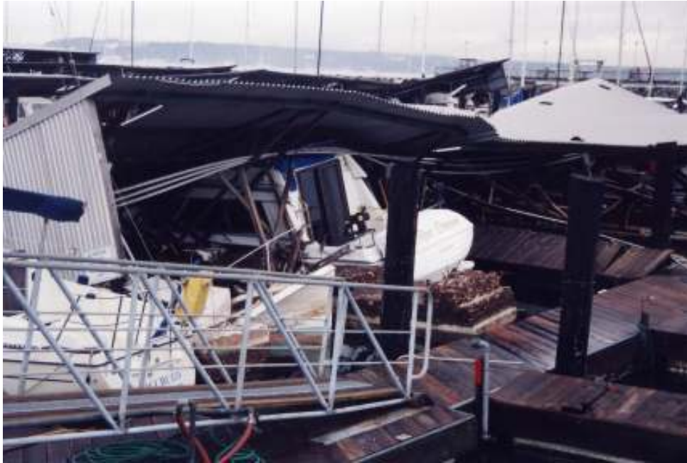
Photograph 2: Dock collapse from winter storms, December 1996. Source: Port of Edmonds
