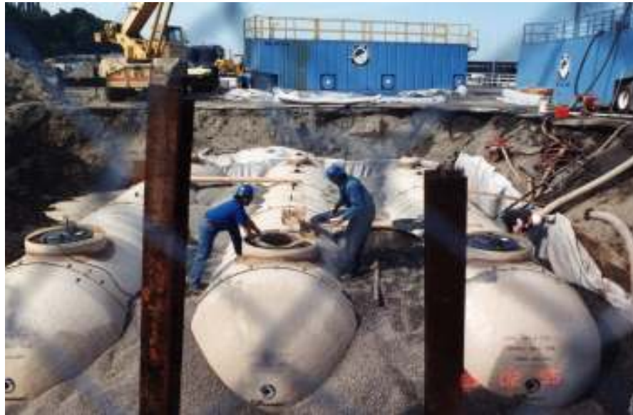
Photograph 4: Double-walled fuel tanks. Source: Port of Edmonds
